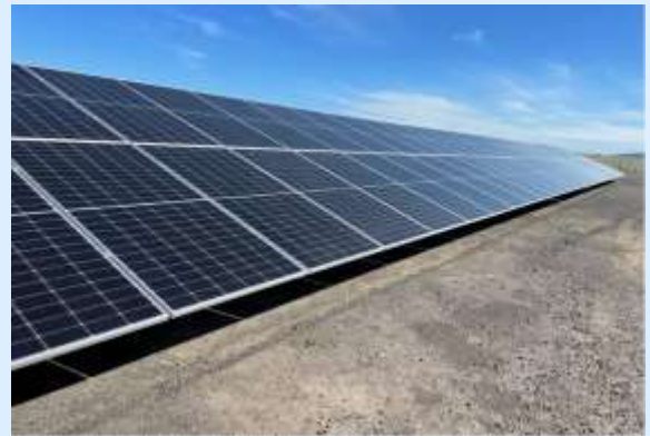
Solar panels at VICSES Fawkner
