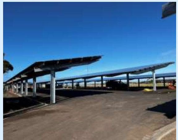
Barwon Prison - Solar power carpark
